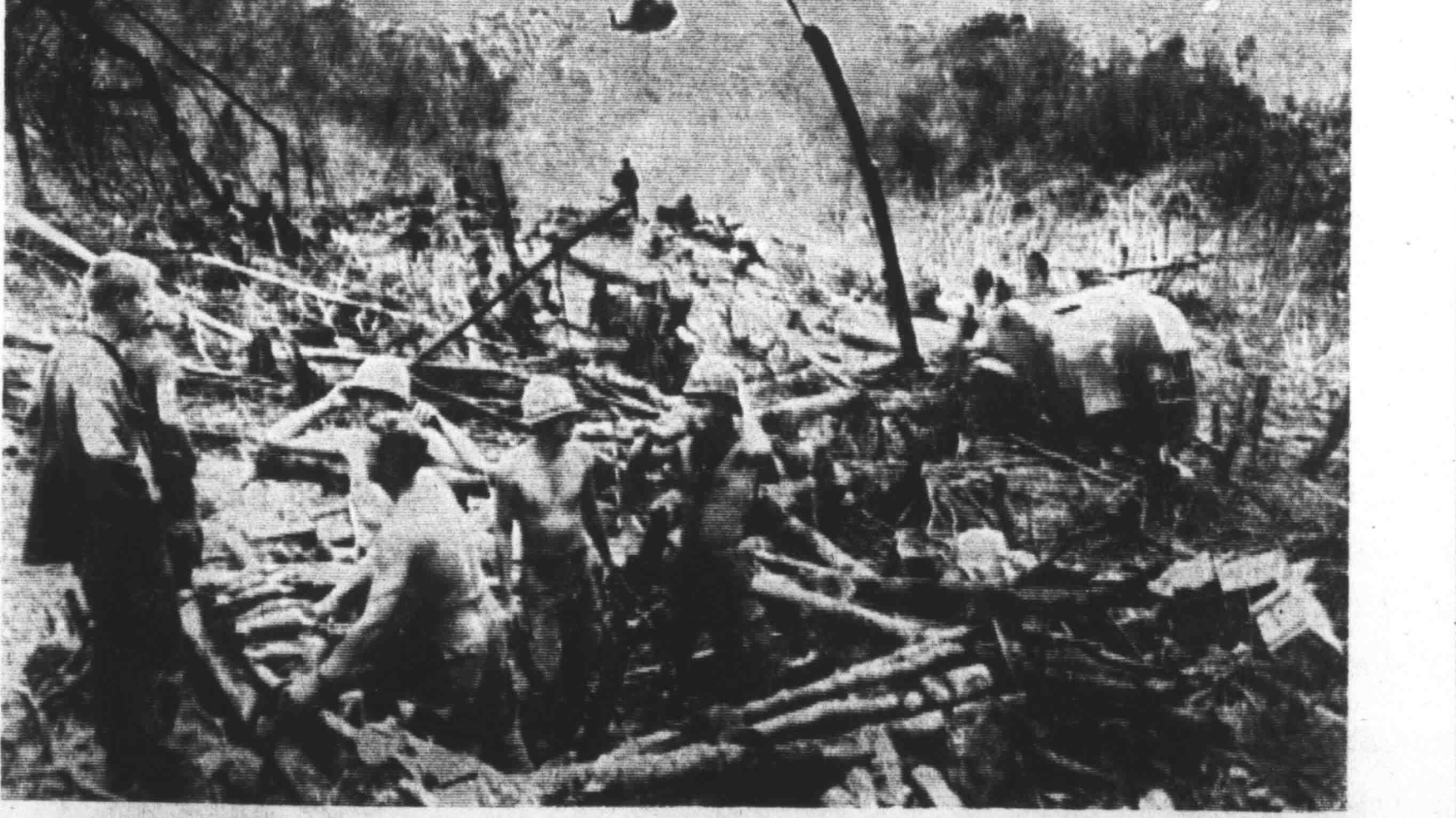
A SHUA VALLEY, SOUTH VIET NAM: U. S. 1st Cavalrymen build mortar bunker after clearing landing area in jungles of Quan Tri Province. Downed helicopter is at right. The joint allied operation is the latest sweep of the valley in an attempt to wipe out the North Vietnamese supply line feeding Communist forces in this strategic South Vietnamese northern frontier.
